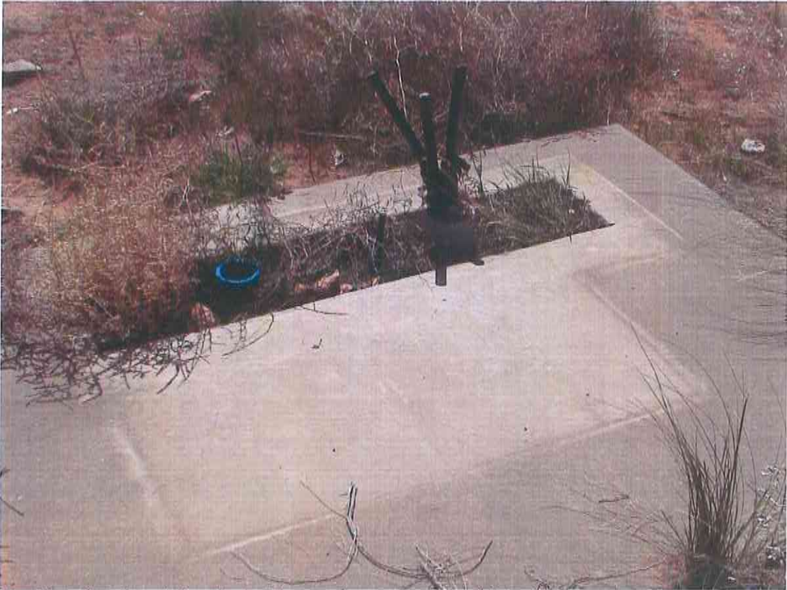
No. 39 – Abandoned electrical wiring on the eastern side of the subject property.
